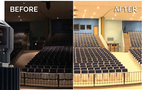
Fairfax High School, Fairfax, Virginia 105 RETRO 500s at 3000K Installed by Artistic Concepts Group
